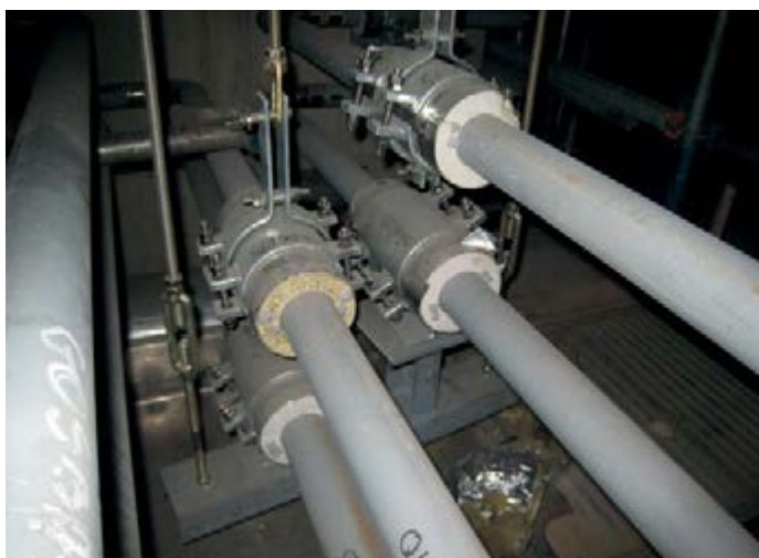
Pipes held in position with cryogenic supports
